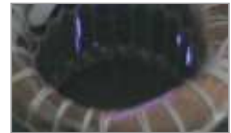
Corona discharge in motor
